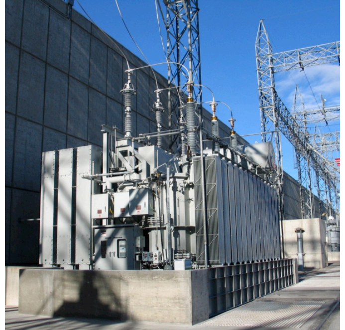
Fig. 4 Application of FO sensor for cooling control on a 240 MVA transformer at GCPUD.
